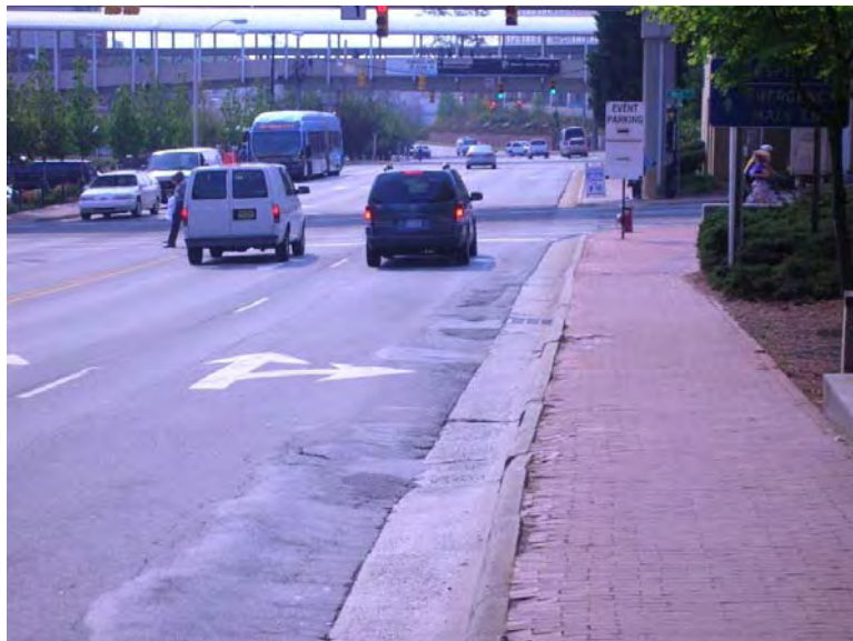
Figure 65. Right lane pavement in the area where bicyclists would ride is also very rough from heavy vehicle/transit use. Both pavement and sidewalks are in need of repair. (Photo by Charlie Zegeer)
