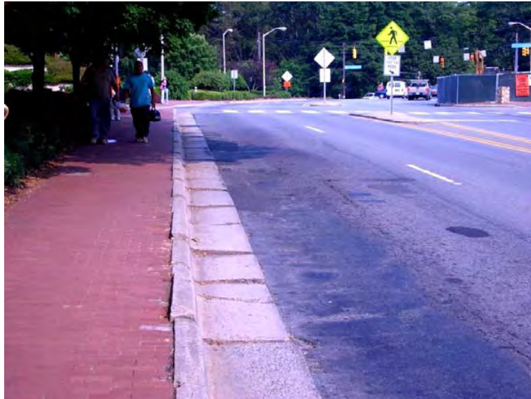
Figure 64. Sidewalk and curbs are extensively damaged in some areas along Manning Dr. Sidewalks on the west end are also immediately adjacent to traffic lanes. (Photo by Charlie Zegeer)
