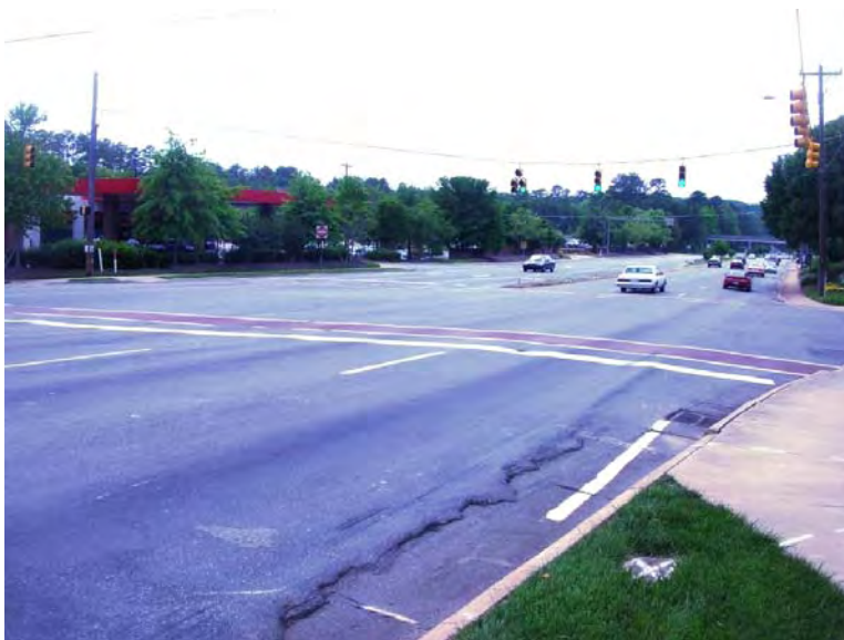
Figure 76. Rough pavement near the right side of the lane is hazardous for bicyclists (near Hamilton intersection).
