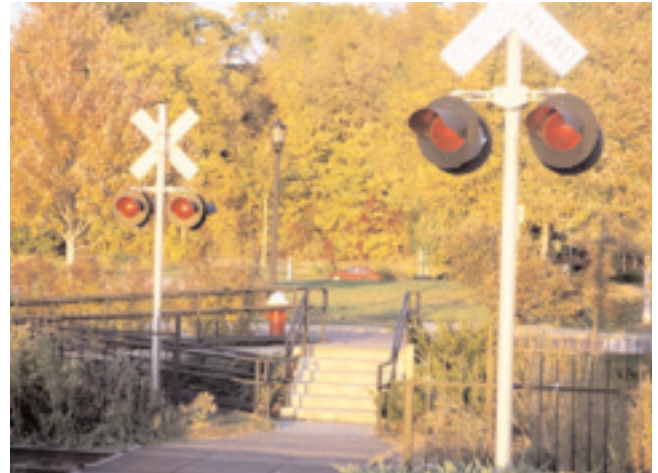
Active warning devices at Burlington Waterfront Bikeway track crossing. Burlington, VT
