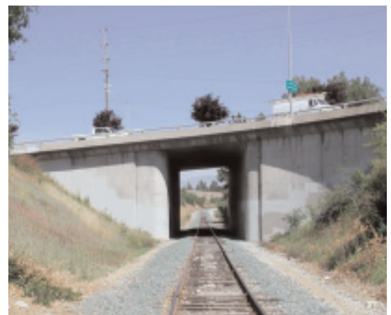
Tunnel along proposed RWT. Trail will be re-routed in this section. Cupertino, CA
